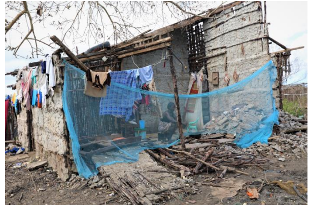
A woman uses a mosquito net to cover the vacant space left by a fallen wall due to Cyclone Freddy. ©UNHCR/Guilherme Chirinda
